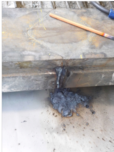
Result of the arc gouging of the track.
